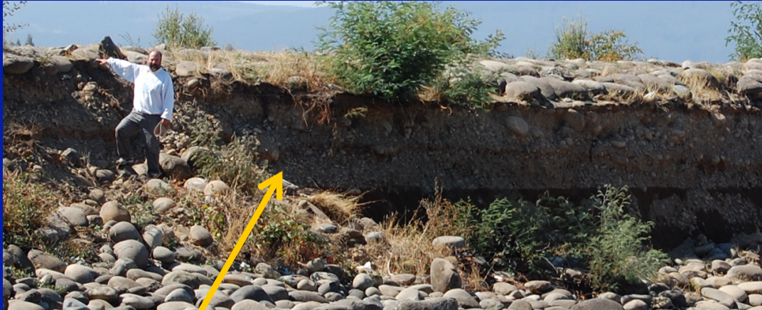
Coihueco Zoned Earth Dam Upstream Slope Failure
